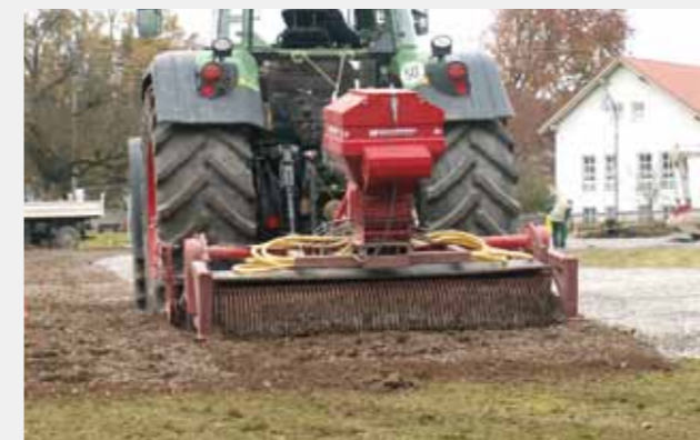
3. Harrowing in the components (60 % by volume ballast and 40 % by volume existing top soil)
