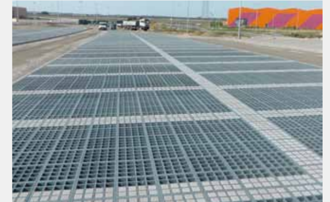
Lay double parking rows continuously and optically separate from each other by a line of stones on the front side. (Mounting during the construction phase)
